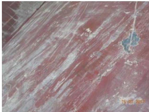
LOWER HOPPER WITH LOOSE PAINT & SCRATCHES
