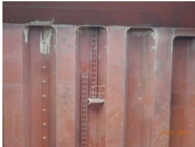
FWD BULKHEAD WITH COAL STAINS
