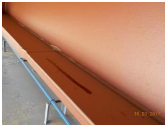
HATCH COVER UNDERSIDES WITH SBM DUST
