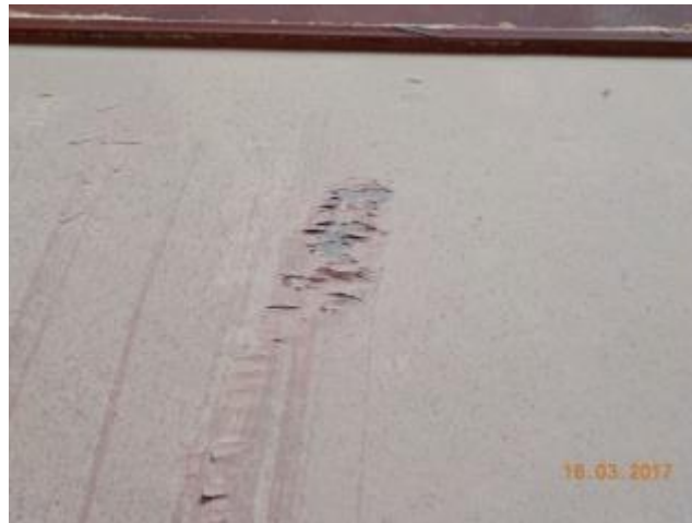
LOOSE PAINT ON LOWER HOPPERS
