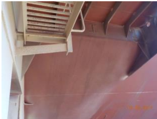
UPPER HOPPERS WITH SLIGHT COAL STAINS
