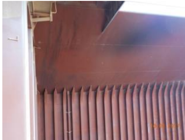
COAL STAINS ON UPPER HOPPER
