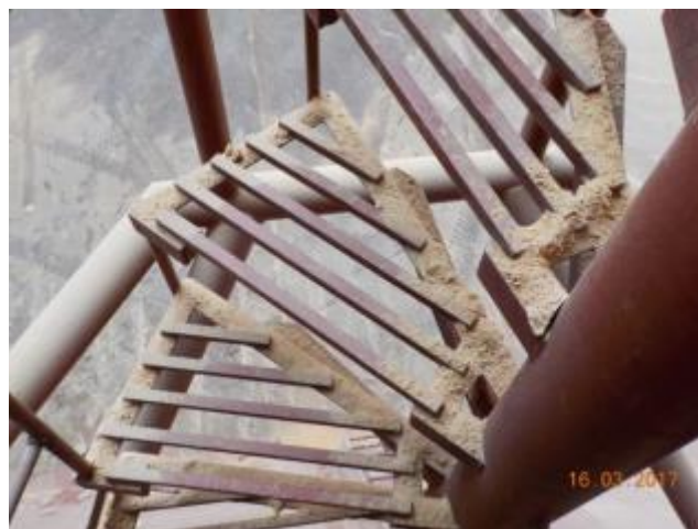
AUSTRALIAN LADDER WITH SBM RESIDUES
