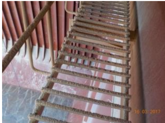
NO. 5 HOLD FWD UNDERDECK PLATFORM WITH SBM RESIDUES
