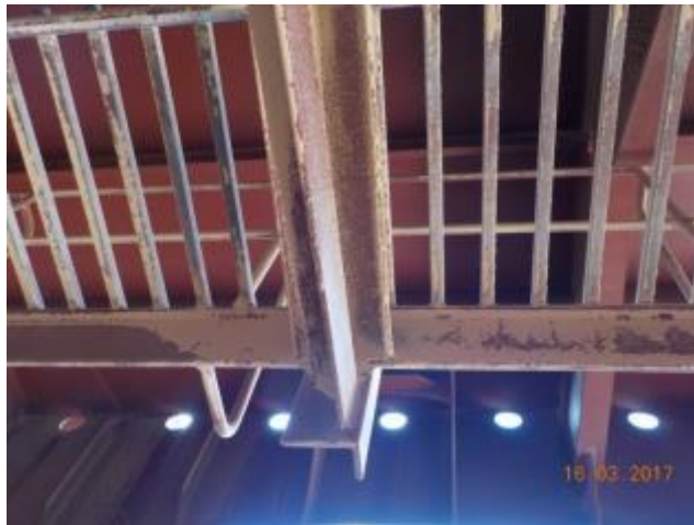
UNDERDECK PLATFORM WITH SBM
