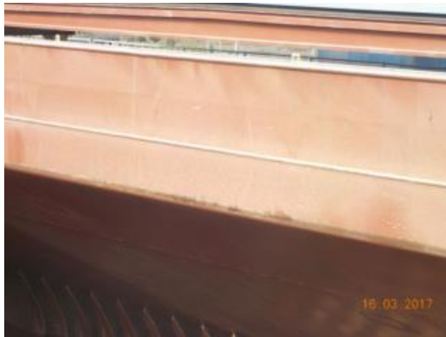
HATCH COAMING WITH GREASE AND SOME LOOSE PAINT
