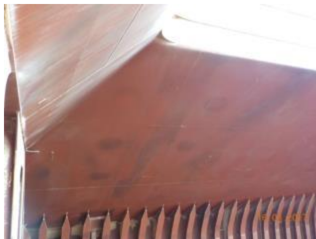
UPPER HOPPERS WITH COAL STAINS
